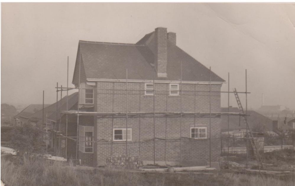
Windy Ridge in the course of construction, and already satisfyingly bigger than its neighbours
